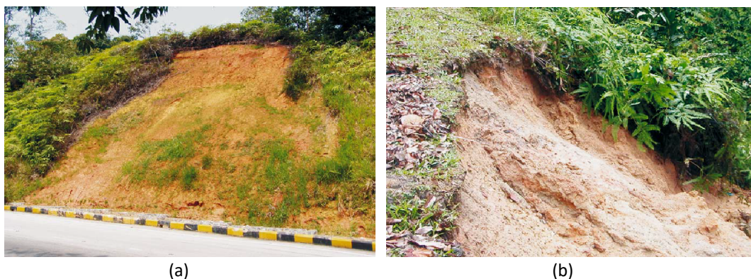
Figure 1: Gully Erosion Features at (a) Fraser Hill and (b) Genting Highlands
